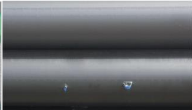
Figure 4 Possible damage caused by handling.
