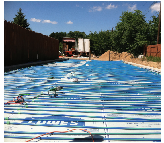
The floor grid for the ABC beer cave is roughly 23 ft x 78 ft with ½-in. Aquatherm Blue Pipe spaced out every 6 in. to provide heating and cooling. The Aquatherm heating iron used to make the heat fusion connections is in the center of the picture. You can see the green couplings in a line to left of the tool.
