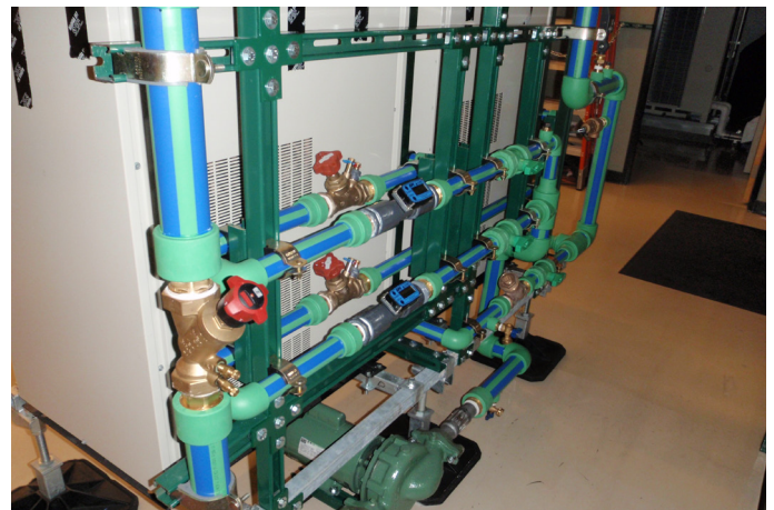
While the Irvine training lab installation doesn't have a large amount of pipe, it does have several connections to valves, pumps and equipment. And the installation didn't have a single leak.
