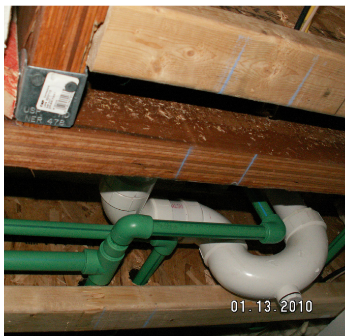
The quick and easy fusion connections allowed the installing contractor, Ripp Construction, to save time on the installation and the job was completed without any leaks whatsoever.
