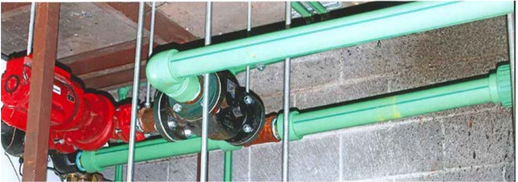
Demand Mechanical used SDR 7.4 Aquatherm Green Pipe®, multi-layer faser (MF) pipe for all of the hydronic heating and domestic hot water/plumbing piping renovations in 2013-14. The piping system is designed for potable and food-grade applications. In this case, it met the operating parameters of 150°F at 100 psi on the domestic hot water side and 180°F at 50 psi on the heating side.
