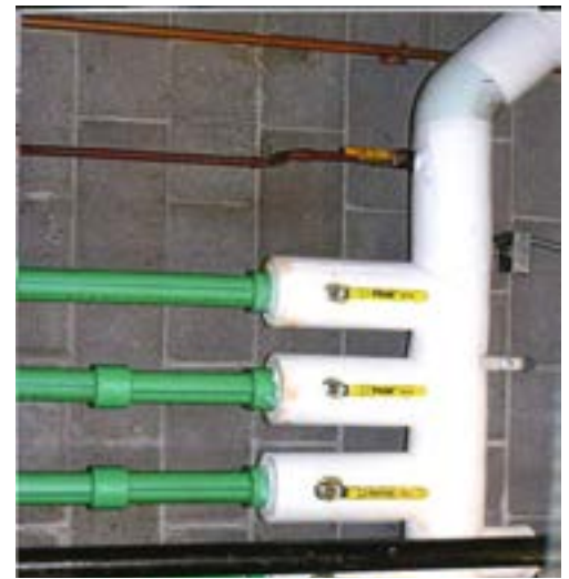
The use of a single pipe material helped facilitate the 2013-14 renovations at the hotel; both the mechanical and domestic water systems were completed in matter of weeks by a small work crew. The Aquatherm Green Pipe® shown here runs in a supply-return configuration and is connected to a Lochinvar water heater.
