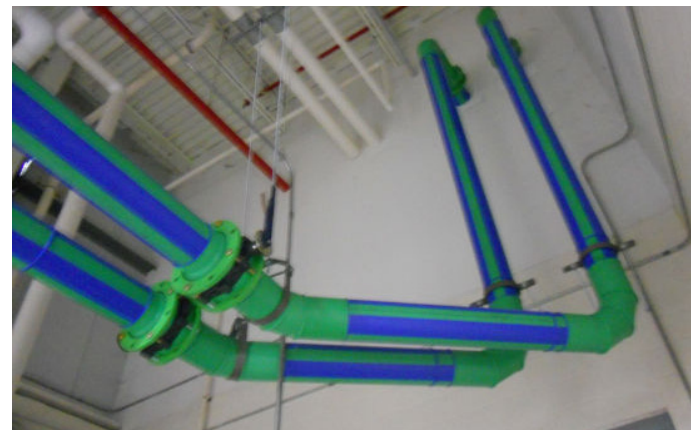
These butt-fused lines serve the boiler testing system. Since PP-R is corrosion proof, plant officials don't have to worry about long-term deterioration of the pipe and problems they'd previously experienced (below).
