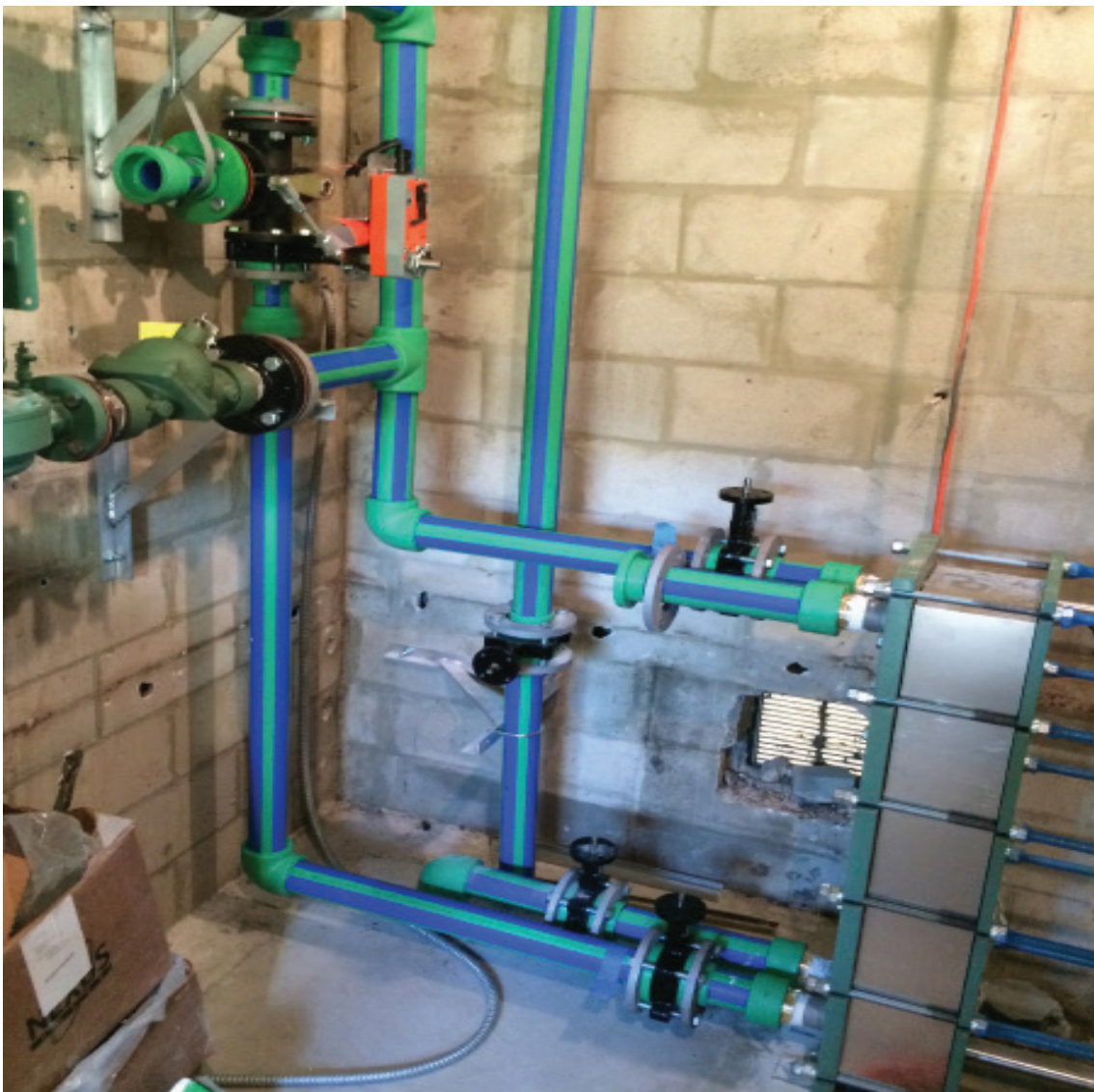
The OCI system included a 25-ton air-cooled chiller and an 8-ft tall, 8-ft diameter ice-storage tank to serve the cooling needs of the facility. A heat exchanger also was installed to separate the ice storage/ glycol loop from the building chilled-water loop serving 11 air-handling units.
