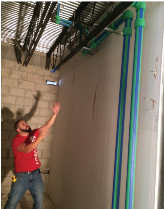
Voila! An OCI engineer-turned-Aquatherm-installer shows off some of the chilled water system's supply and return lines.
