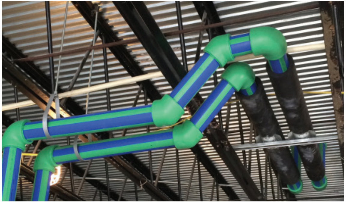
Based on the itemized bids they had received from several mechanical contractors, OCI Associates saved approximately $85,000 in material and labor costs by using Aquatherm Blue Pipe instead of steel for their mechanical system.
