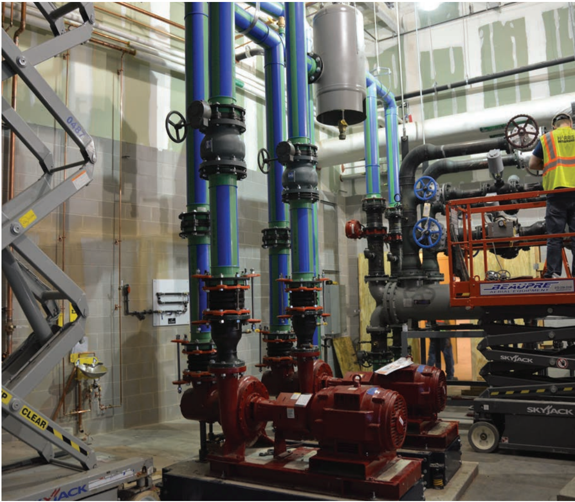
The mechanical room for the field heating system features large diameter Aquatherm Blue Pipe connecting to Bell & Gossett, ABB and other mechanical equipment.
