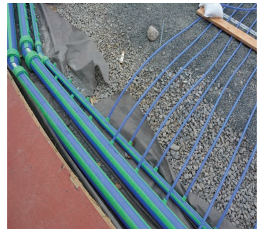
The Aquatherm Blue Pipe manifolds that run around the field perimeter, with coiled Blue Pipe connecting to them via fusion outlets.
