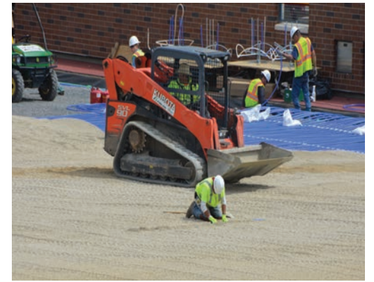
A skid-steer grades the sand layer that covers the Aquatherm Blue Pipe coil grids that heat the field.
