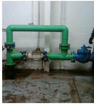
After seeing PP-R perform so well for three years, Tri-State installed it for its six-inch main line.
