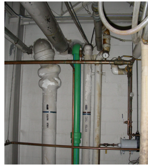
The soft water main runs from the three water softeners in the boiler room to the tunnel washers at the back of the facility. It is a run of approximately 400 feet.
