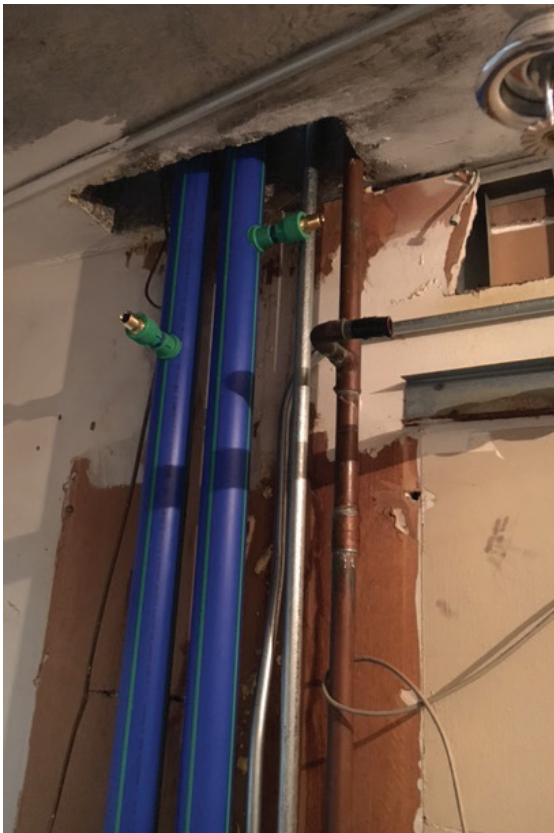
Aquatherm pipe was able to be heat fused and installed in tight quarters without welding or open flame, which was extremely important in an occupied building.
