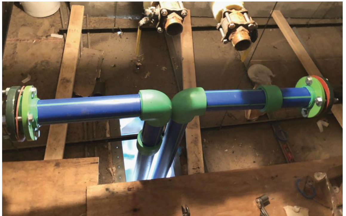
At this project, Aquatherm Blue Pipe® replaced an old and leaky system composed of steel and copper pipe.
