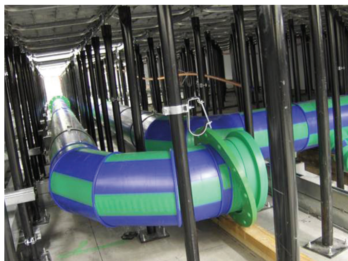
Large diameter Aquatherm pipe in place as part of the cooling system for the supercomputers at Lawrence Livermore National Laboratory.
