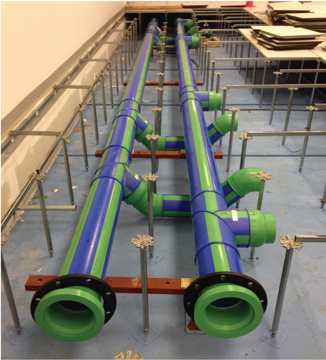
Aquatherm pipe being installed at the TierPoint Jacksonville data center in 2014.
