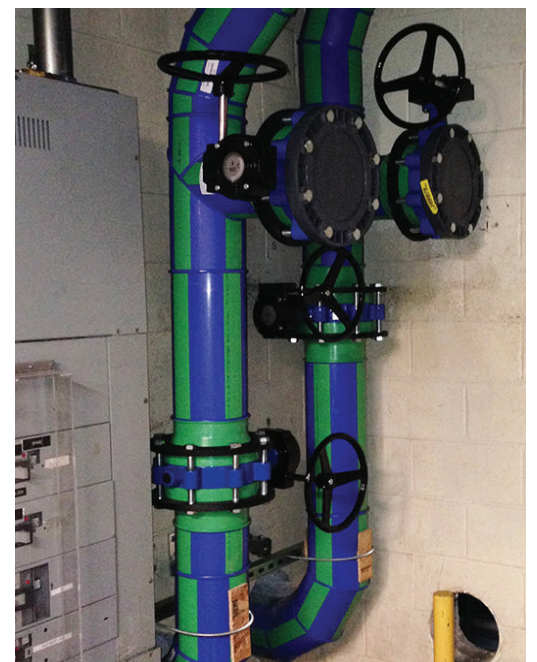
Aquatherm pipe has been helping ensure the safety of clients' data at this data center for more than six years.
