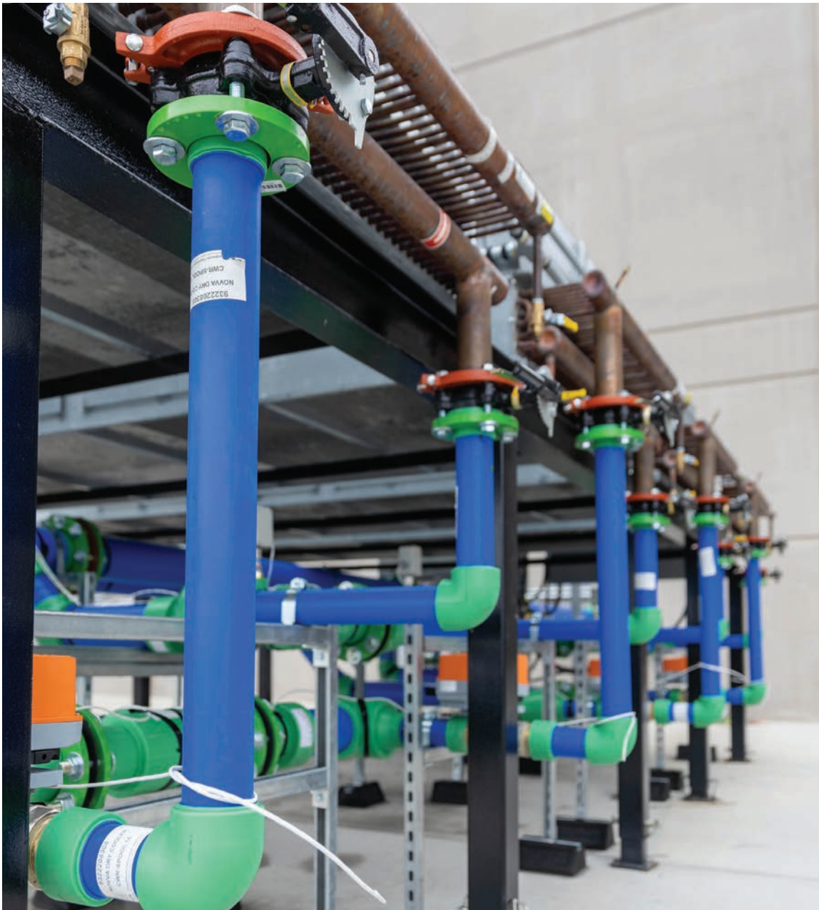
More than 4,400 feet of Aquatherm pipe was installed during the first construction phase of this project.
