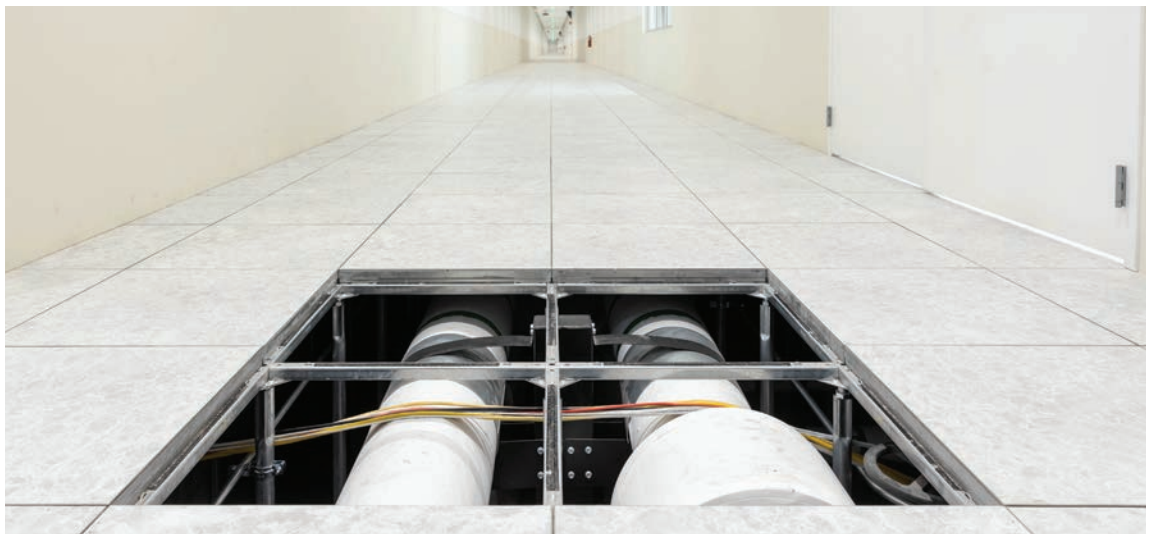
Aquatherm's BIM and Scan-to-Fab services were key to a smooth installation of the underfloor cooling system.
