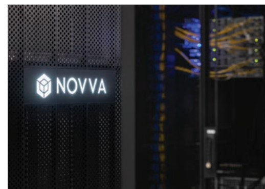
The main entrance of the Novva data center and headquarters in Utah.
