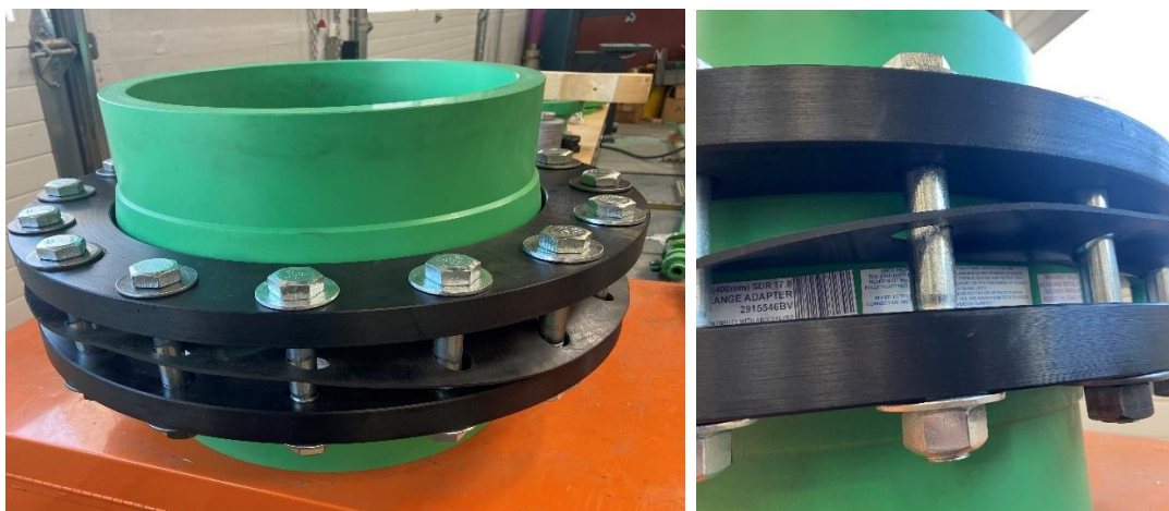
Figure 1 – Photos of installed bolt/nut/washers on new rings using Aquatherm flange-to-flange and 1/8-in EPDM gasket
