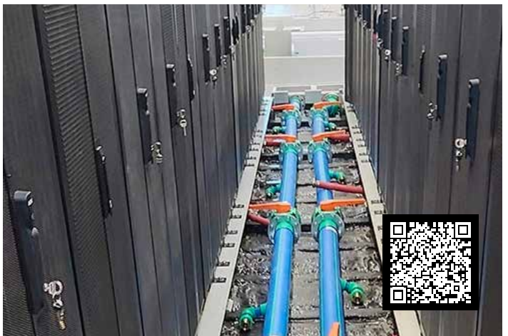
PROJECT Modular Data Centers Cooling System
